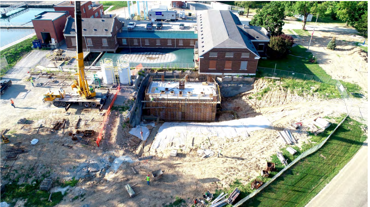
Figure 5: Photo looking from the north towards the project site taken in early August.
