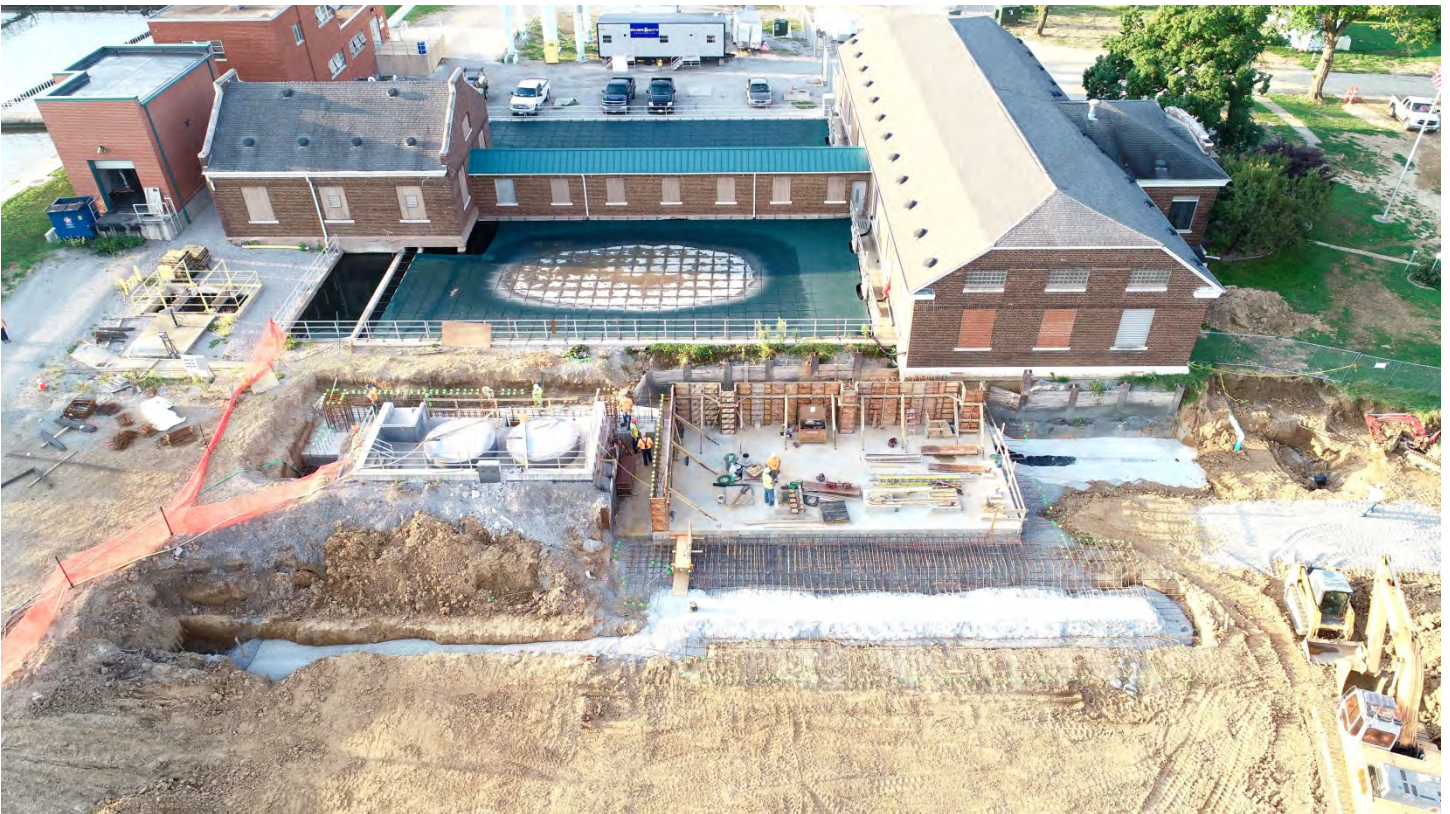
Figure 6: Photo looking from the north towards the project site taken in early September.
