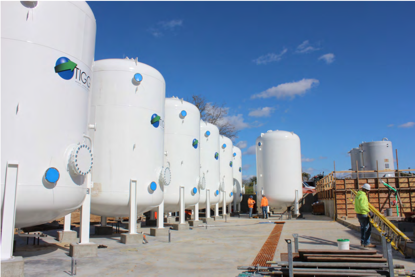
Figure 9: Picture after the eighth GAC vessel was set into place on the afternoon of October 22, 2019.
