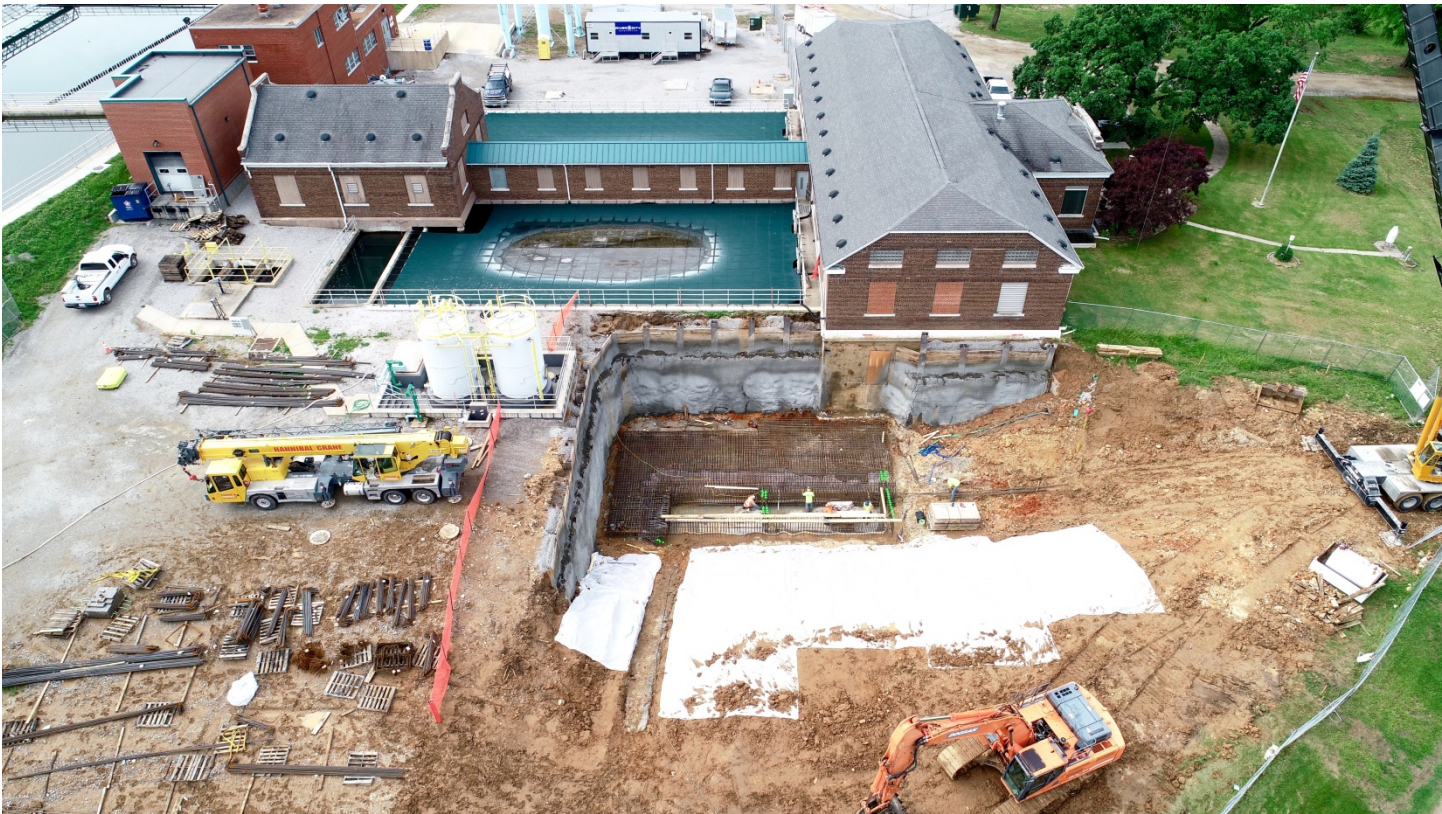
Figure 3: Photo looking from the north towards the project site taken in early June.
