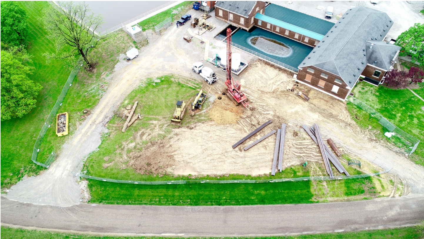
Figure 2: Photo looking from the north towards the project site taken in early May.
