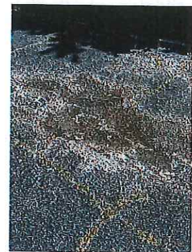
Figure 2 – Deteriorated Surface Area/ Evidence of Prior Ponding
