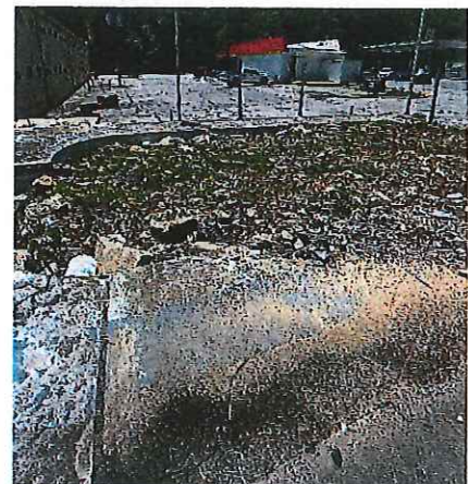
Figure 7 - Unsecured Swimming Pool filled with Rock and Debris
