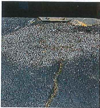
Figure 1- Deteriorated Surface Area
