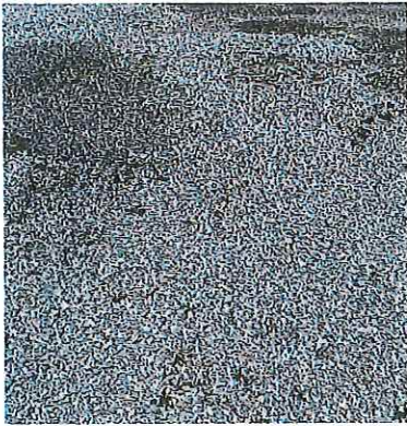
Figure 4 – Deteriorated Surface Area
