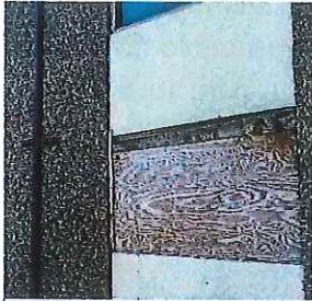
Figure 5 – Boarded Up Windows
